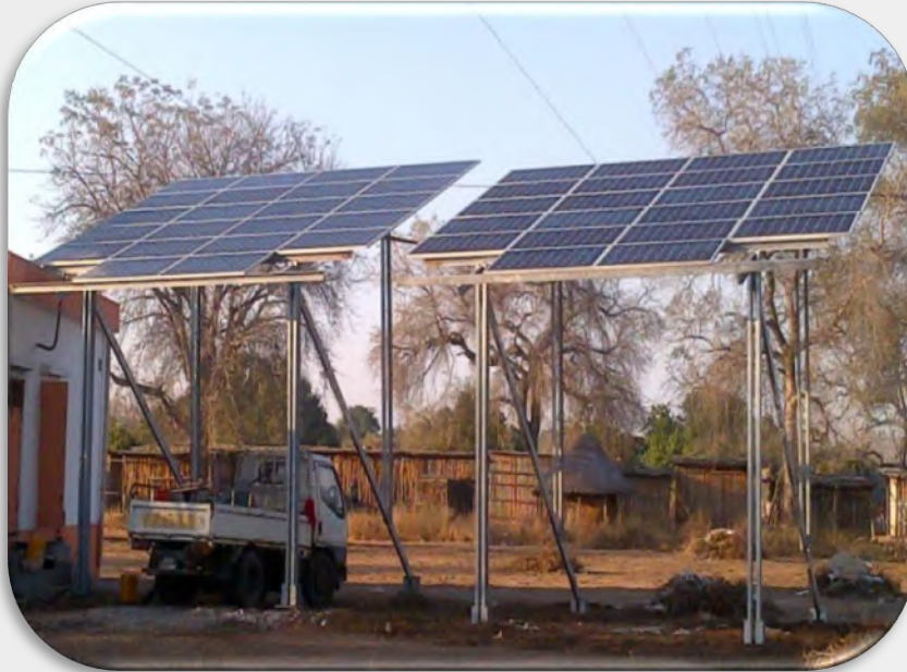
500kw Solar Power PV Station Mozambique year 2015
