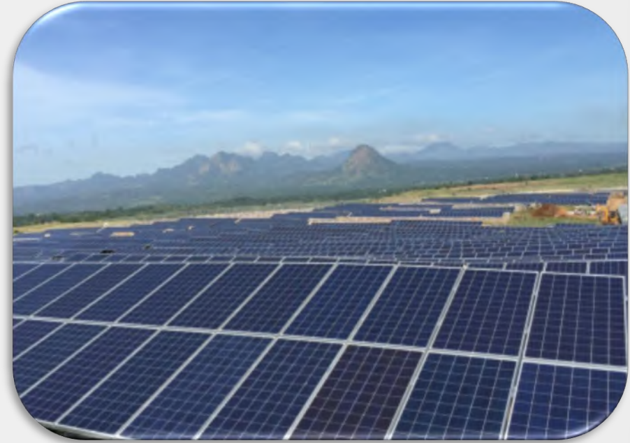
14.5MW Solar Power PV Station Philippines year 2015
