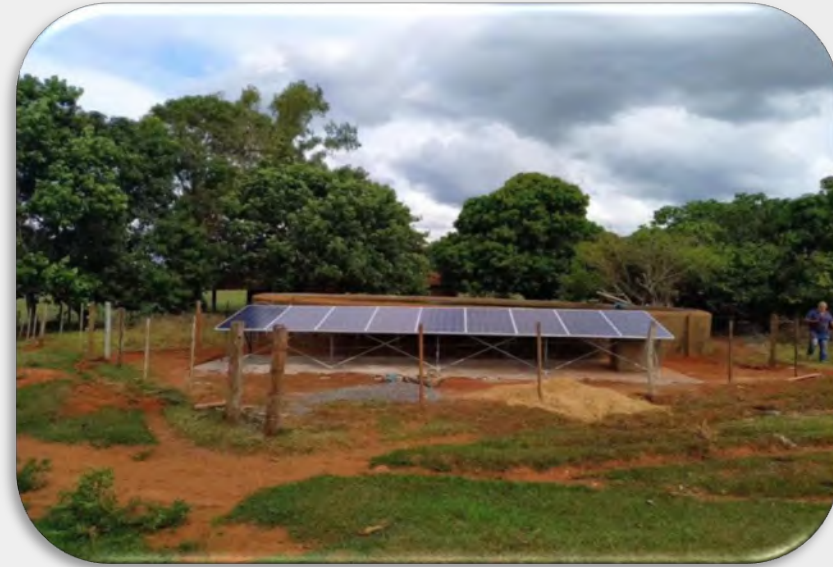
200kw Ground Project Philippine year 2016
