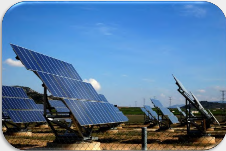
2.8MW Power Plant Spain year 2012
