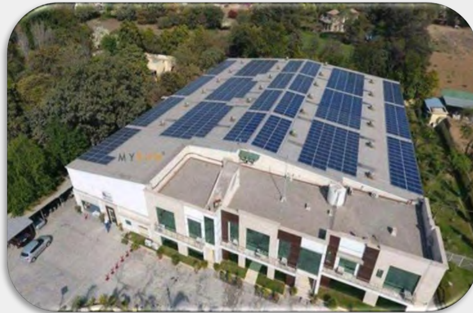
600kw Roof System Colombia year 2016
