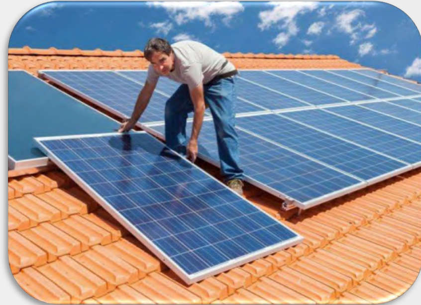
800kw Roof System Netherlands year 2014
