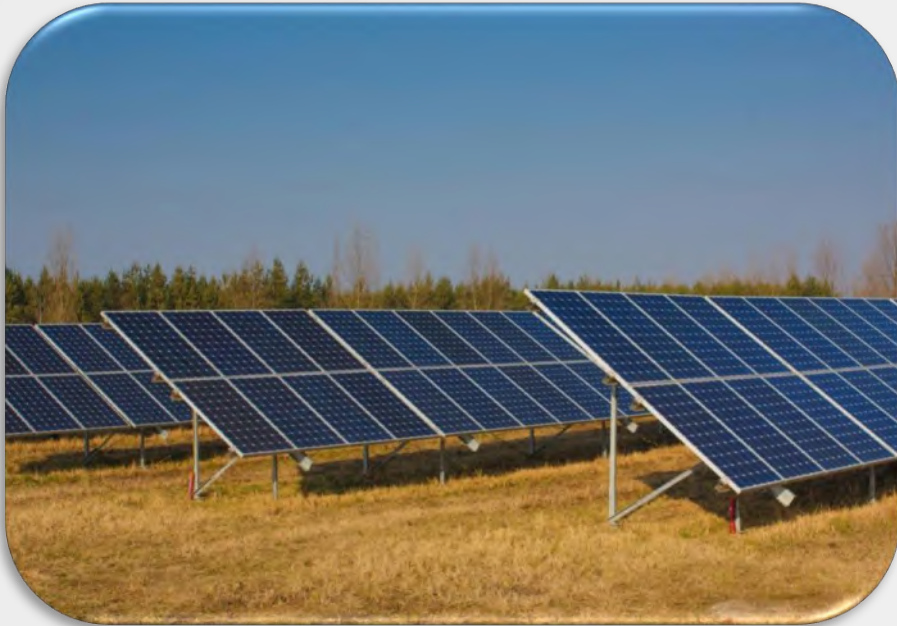
3.5MW Solar Power PV Station Czech year 2016
