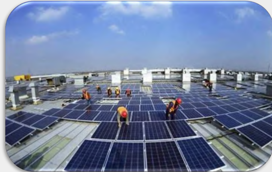
2MW Power Plant Portugal year 2018
