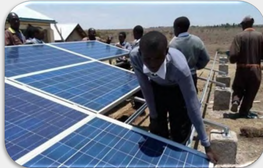
800kw Solar System Angola year 2018
