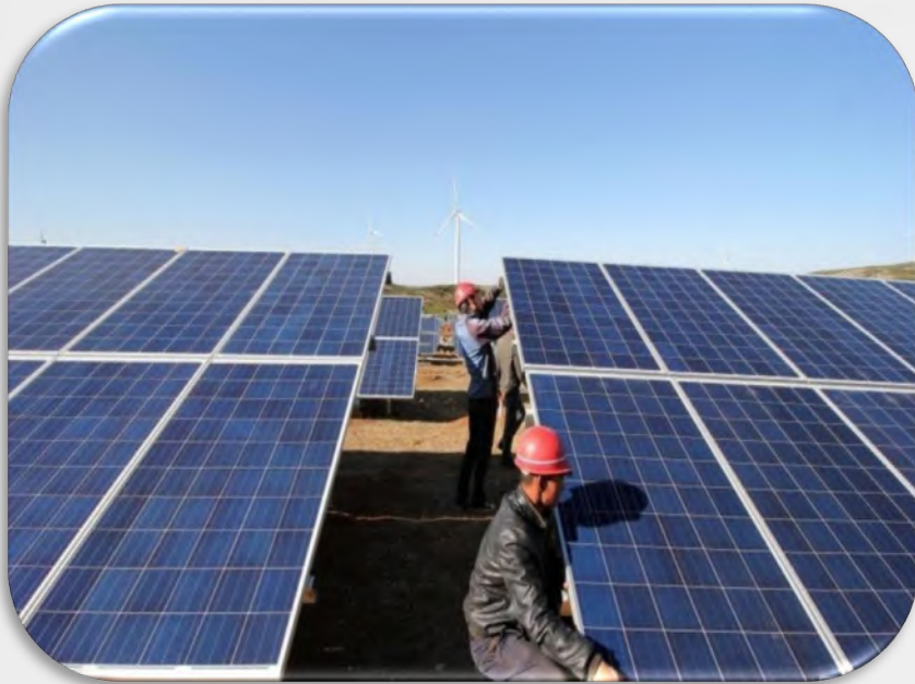
100MW Bao Ying Solar PV Power Project Jiangsu Province ,China year 2016
