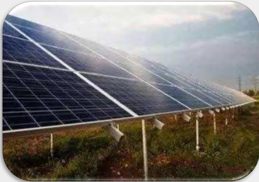
5MW Power Plant France year 2012
