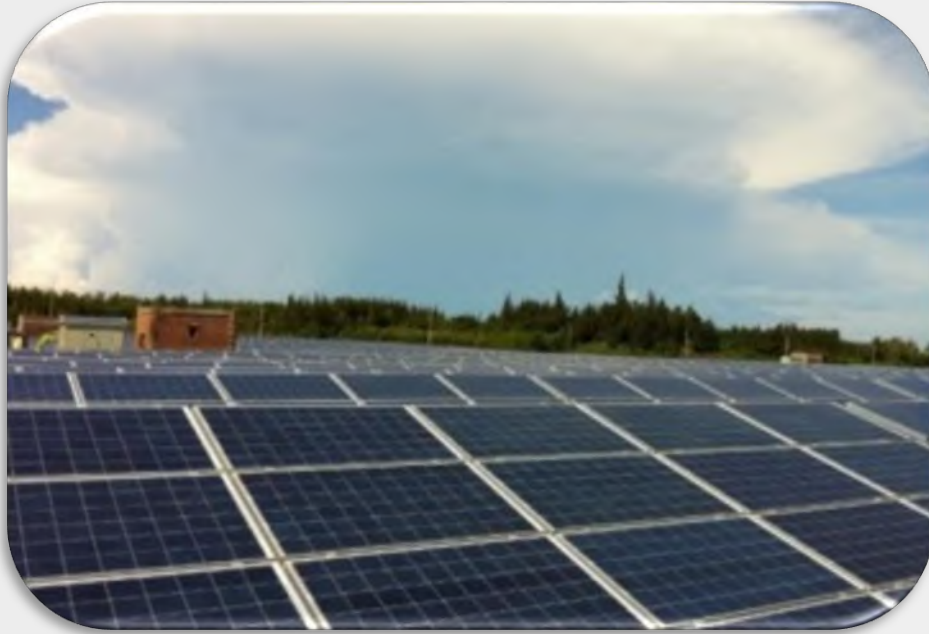
2MW On-grid Solar Power Project Malaysia year 2014
