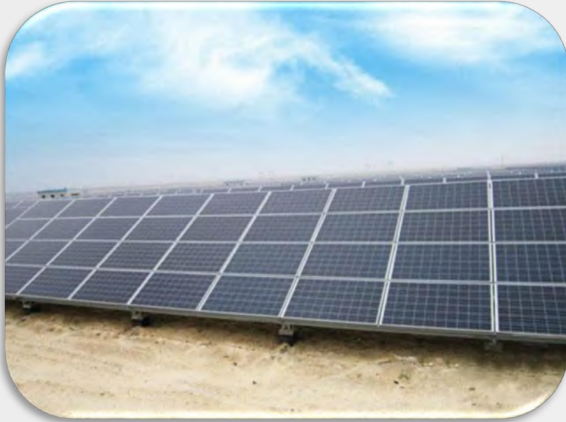
100MW On-grid Solar PV Power Generation Project Gansu Province, China year 2013
