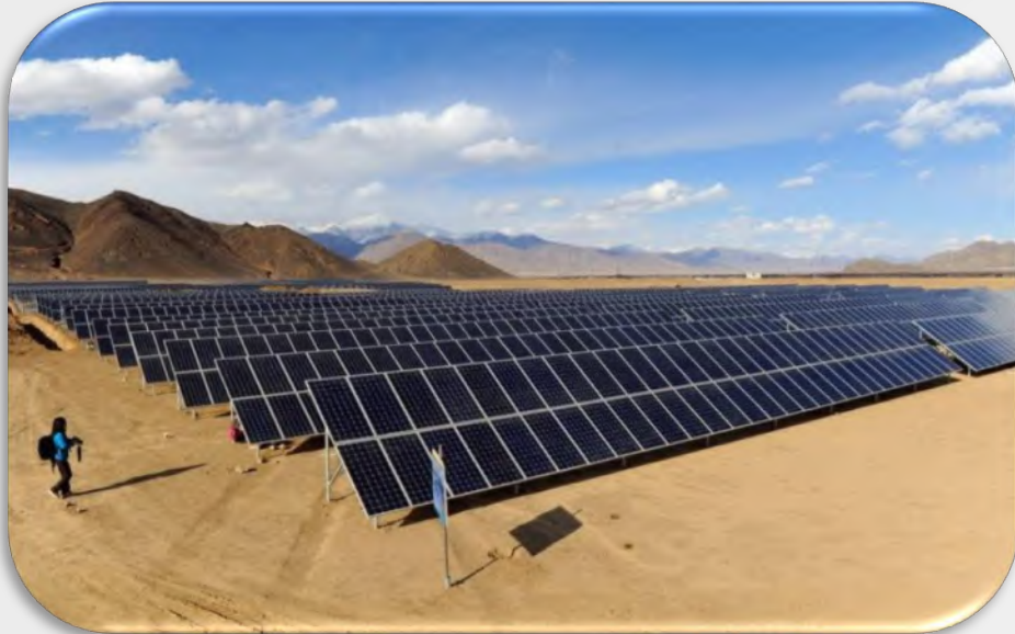
15MW Power Plant Brazil year 2017
