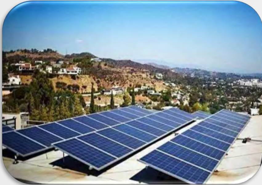
500kw Power Plant Egypt year 2017
