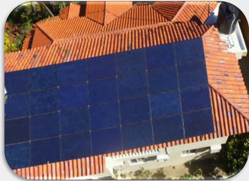
500KW Solar Power PV Station Dominica year 2016
