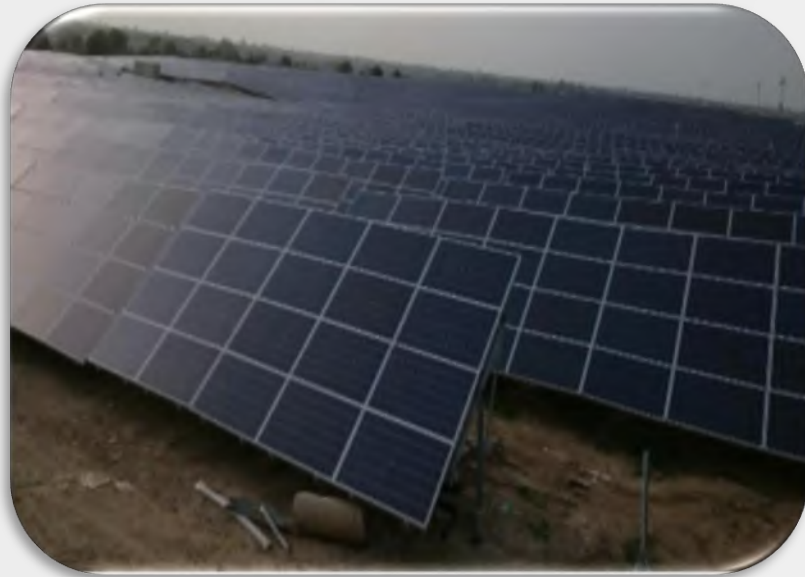
25MW On-grid Solar Power Project Utter Pradesh, India year 2015
