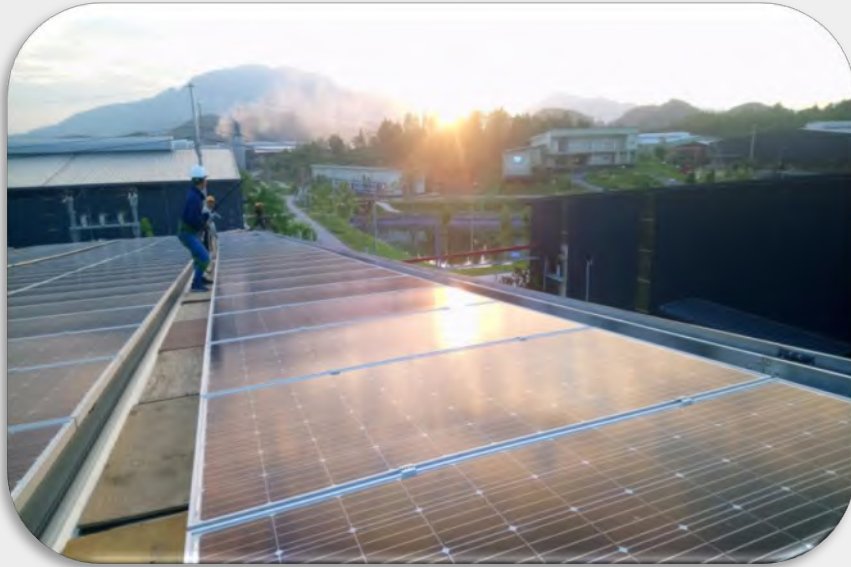
1MW Roof Project Vietnam Year 2019
