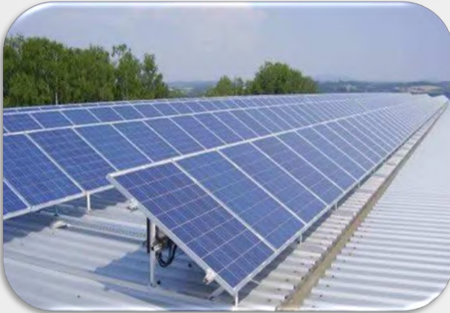
3MW Solar Power Plant Hungary year 2019
