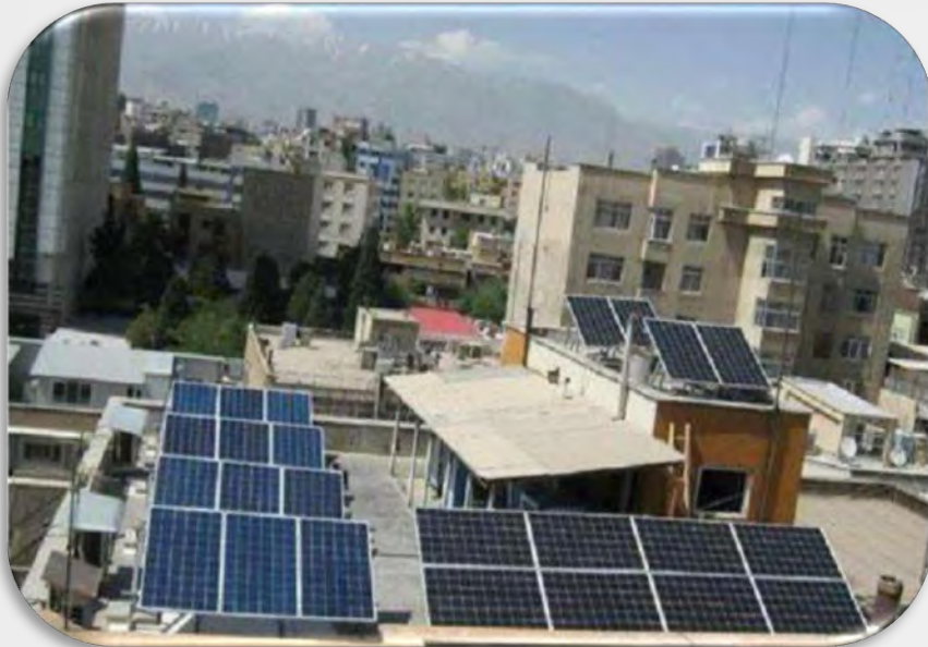
300kw roof system Iran year 2015
