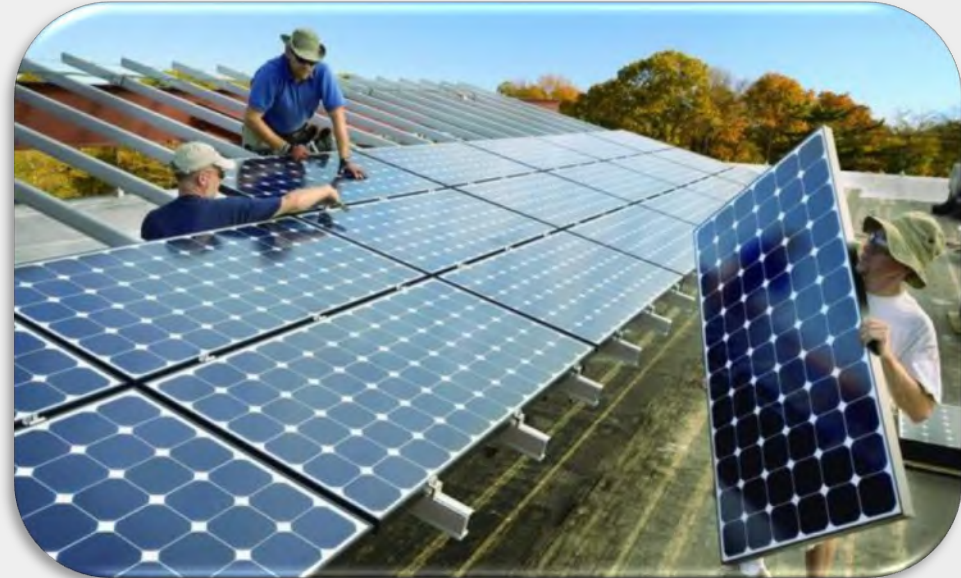
800kw Power Plant Chile year 2016
