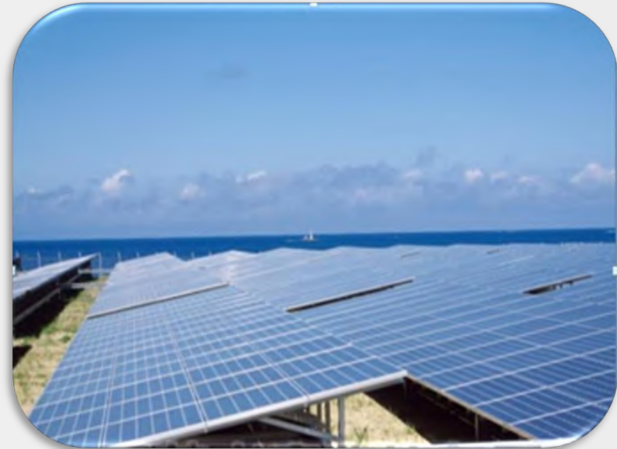
5MW Ground Power Plant by seaside Japan year 2012
