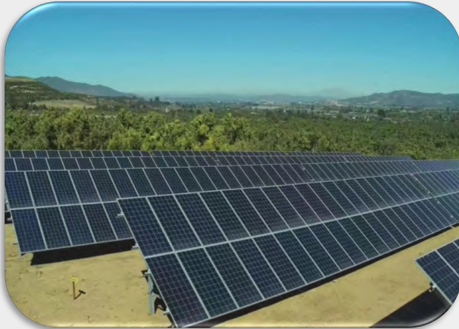
2MW Power Plant Thailand year 2012
