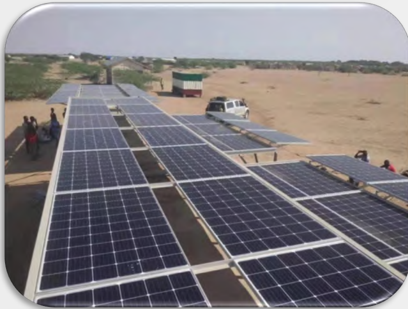
1MW Solar Power PV Station Kenya year 2015
