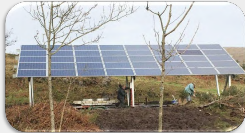
100KW Solar System Cork 2018
