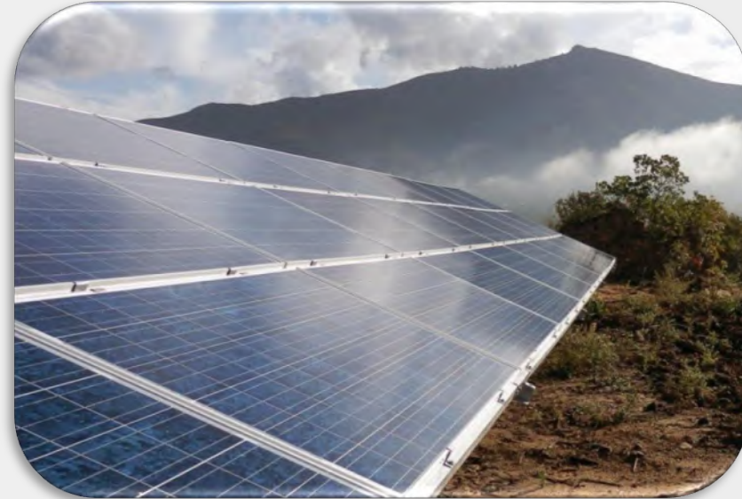
4.5MW Solar Power PV Station Corsica 2014
